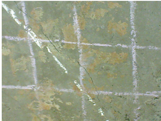
Fig. 8 Diagonal cracking in deep beam
