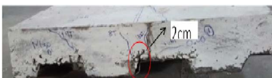
Fig. 9 Slip behaviour for slab 0°
