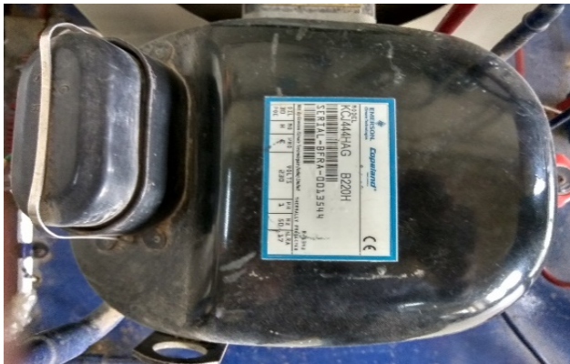
Fig.2 Compressor of the VCRS.
