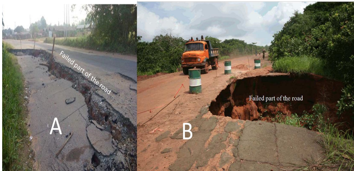
Fig. 2 (A & B) Pictures showing road infrastructure failure caused by flooding and erosion from [16] and [20]
